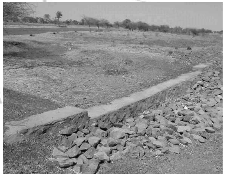
A bund to harvest rain water in Surodi village, Maharashtra, constructed as part of the Watershed Development Program.
